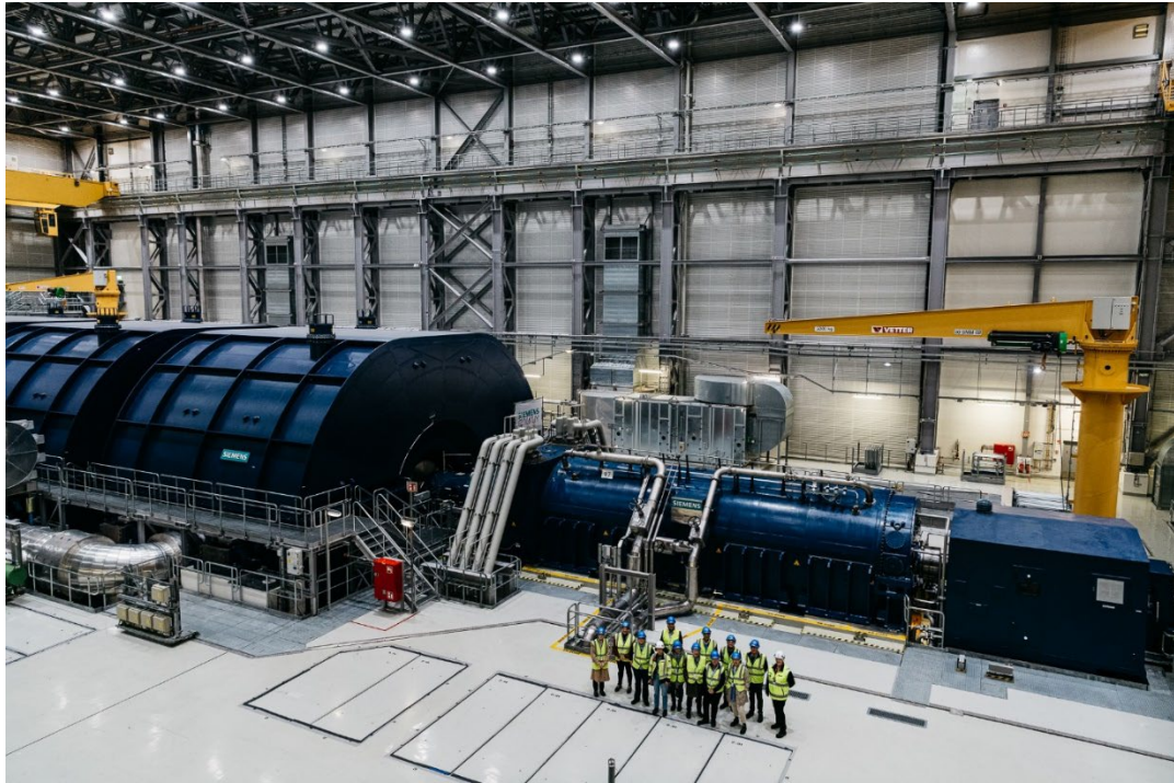
Visit of the large turbine building of Olkiluoto 3 (photo credit: TVO / T. Karjanlahti)
